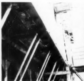
MADE IN SECTIONS. —View of edge of house section, above catwalks, made in sections to be laid in horizontal sills bolted to engine skid bases.
